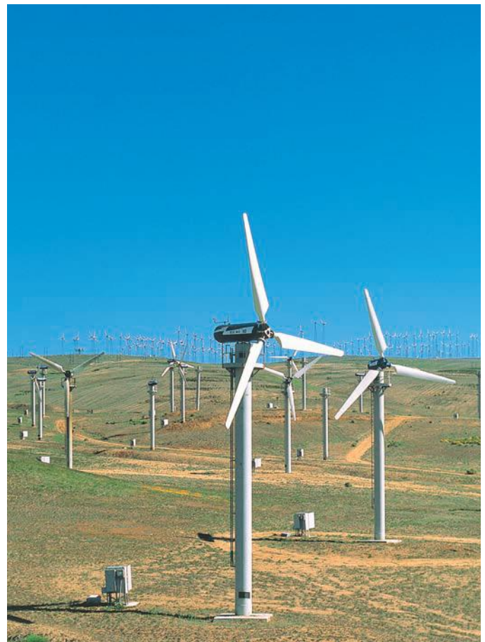
Figure 21.31 Wind generators in the USA. On otherwise unproductive land or offshore, these generators make an increasing contribution to the electricity supply.
